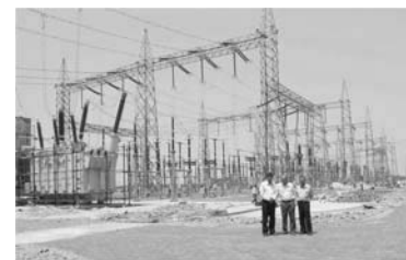
Fig. 20 The substation of Powergrid Corporation of India (near Kolkata, India) where the FBG temperature sensors have been installed. In the photograph, the author is with Dr. Tarun Gangopadhyay and Mr. Kamal Dasgupta. [Slide Courtesy: Dr. Gangopadhyay and Mr. Dasgupta, CGCRI, Kolkata].
