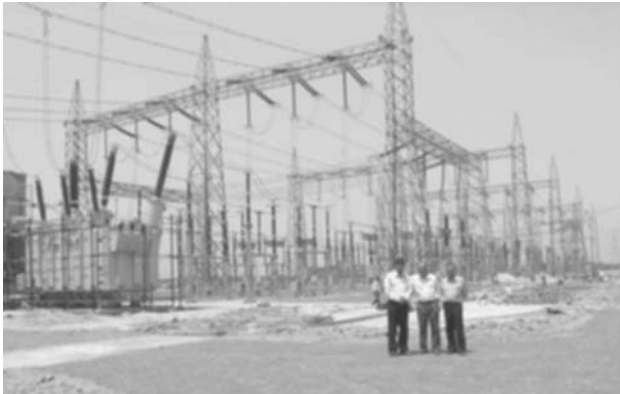
Fig. 15.15 The substation of Powergrid Corporation of India (near Kolkata, India) where the FBG temperature sensors have been installed. In the photograph, the author is with Dr. Tarun Gangopadhyay and Dr. Kamal Dasgupta of CGCRI, Kolkata. [A color photo appears as Fig. 20 in the prelim pages]
