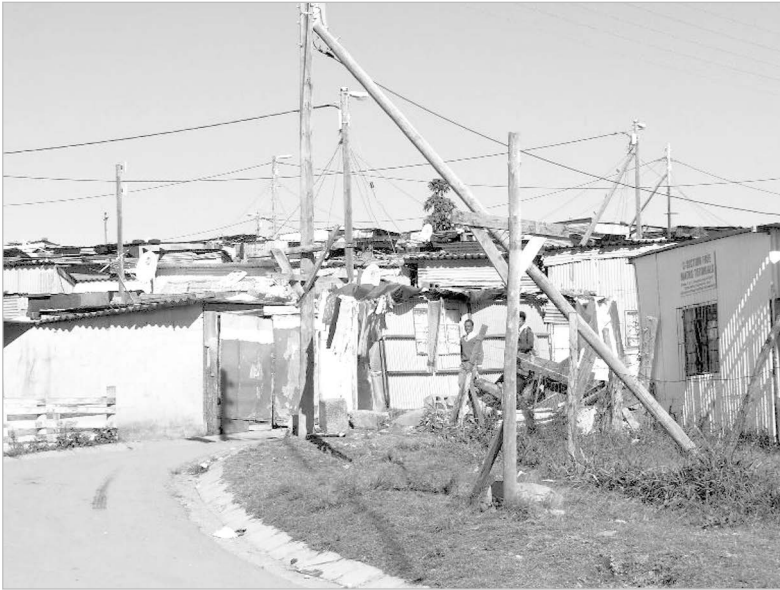
Figure 7: Electrification of informal settlements in Duncan Village.
